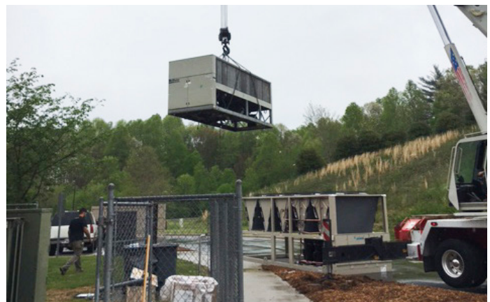
The existing chiller is removed to make way for a new Daikin Trailblazer air-cooled chiller that could save $48,000 in energy costs over seven years.
