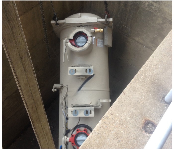
Limited access to a lower-level mechanical room facilitated carefully planned coordination to overcome a challenging installation.
