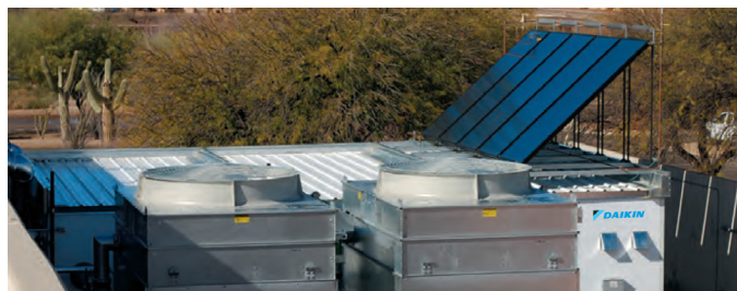
The Modular Central Plant includes solar panels used to heat domestic water, further increasing energy costs savings.
