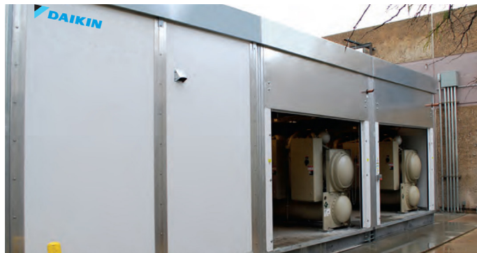
Two 300-ton Daikin Magnitude chillers and cooling towers replaced Pima's outdated chilled water central plant.
