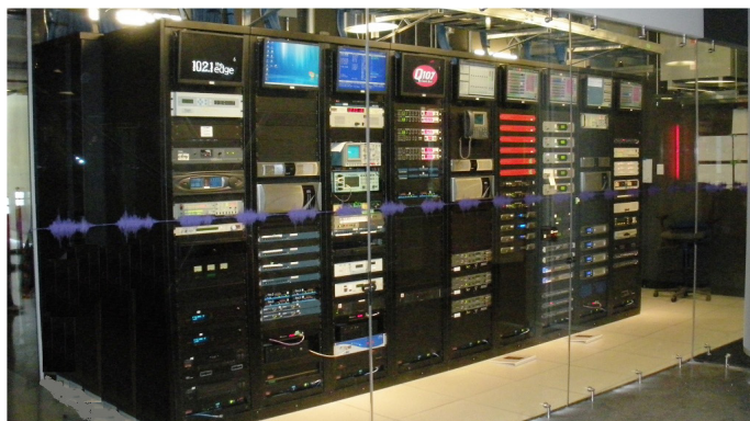
The Daikin chillers supply mission-critical cooling to many locations within the building, including areas like this data center.
